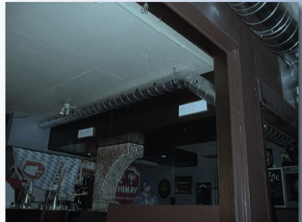
Exposed Duct with Drilled Outlets
